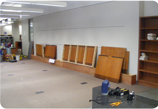
The area between the Public Service Desk and the Fiction Movies and Music desk during construction.
